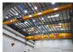
15T & 7.5T X 23M Overhead Crane
