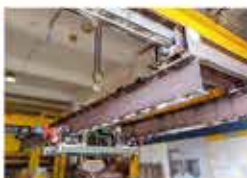
10T Underhung Crane
