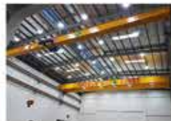
15T & 7.5T X 23M Overhead Crane
