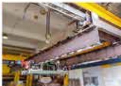
10T Underhung Crane
